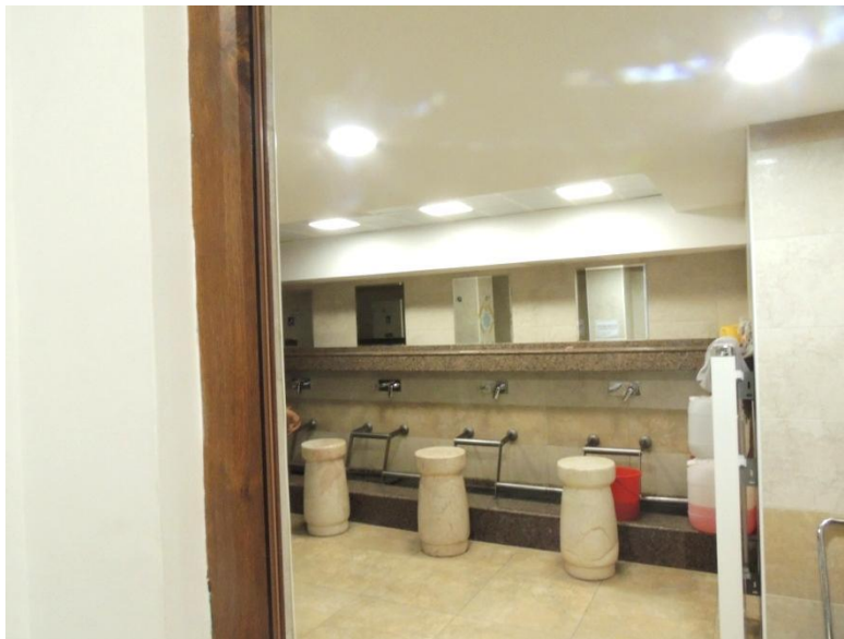
Fig. 73 Kocatepe Mosque, restroom and ablution taps.
